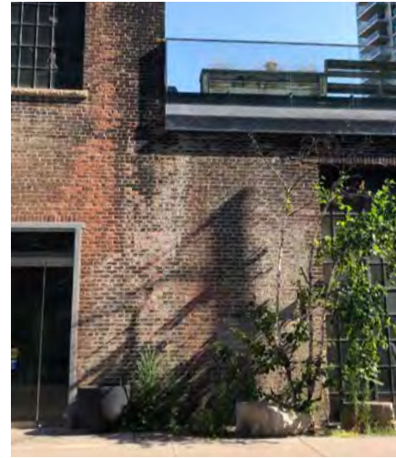
Figure 74. Detail of facade efflorescence (ERA, 2023).
