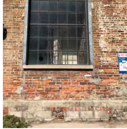
Figure 73. Detail of staining beneath the stone sill (ERA, 2023).
