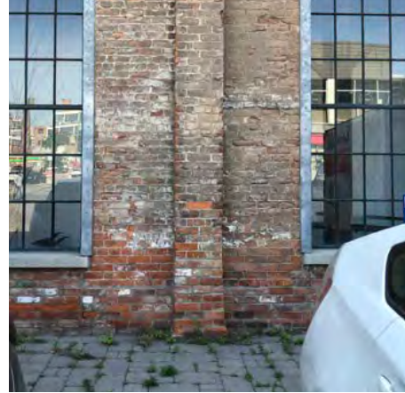
Figure 76. Detail of spalling and joint deterioration (ERA, 2023).
