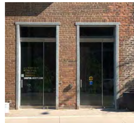
Figure 75. Entrance doors surrounded by galvanized steel plates (ERA, 2023).
