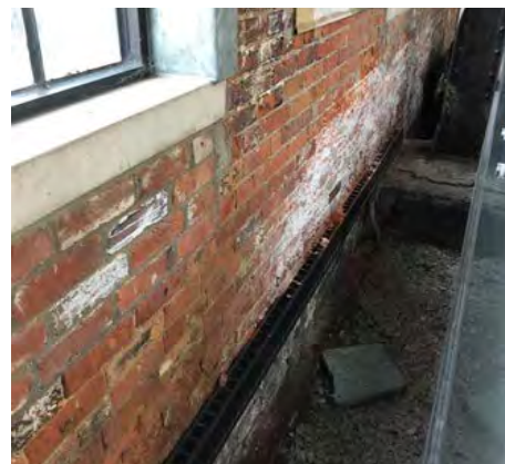
Figure 85. Interior detail of localized brick spalling at-grade (ERA, 2023).
