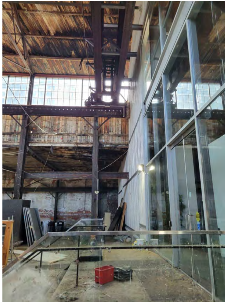
Photo 7: Existing gantry crane located just south of grid line 7
